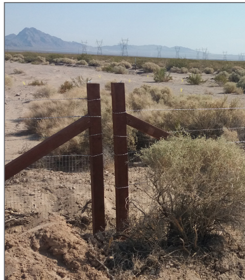
Wooden fence posts were used in select areas to avoid interference with underground communication lines.
