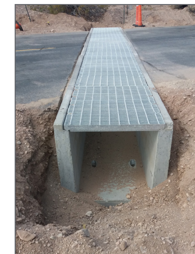
Culvert constructed along Eldorado Valley Drive that will allow for habitat connectivity between the north and south sides of the road.
